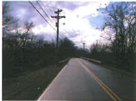
Narrow bridges create safety issues for non-motorized roadway users. Therefore, all new bridges should include accommodations for both bicyclists and pedestrians.
