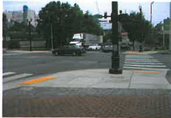
Curb ramps should be parallel with the direction of pedestrian travel, which requires two ramps per corner. Diagonal ramps tend to direct pedestrians toward the center of the intersection, which can be hazardous for sight-impaired pedestrians.
